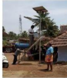
Rural Energy Systems
